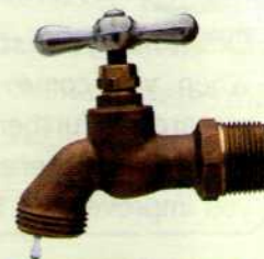
tap is leaking
